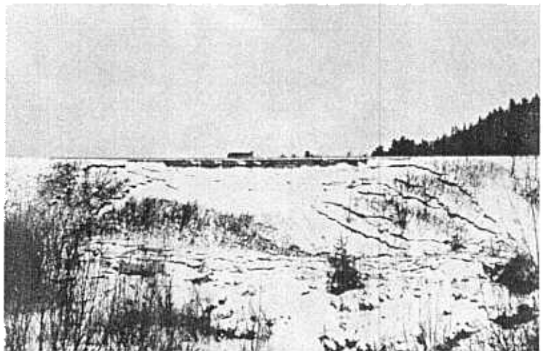
Figure 4: Overall view of embankment failure (60 m long) near Ste-Anne-de-Baupré (Québec).
