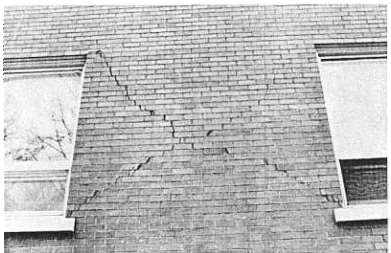
Figure 2: Diagonal cracks in brick wall of Notre-Dame Pavilion, Saint-François-d'Assise Hospital, Québec City (Québec).
