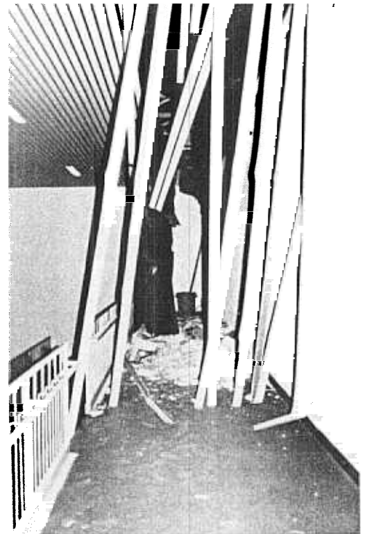
Figure 1: Debris from fallen masonry blocks in Dominique Racine Secondary School, Chicoutimi (Québec).
